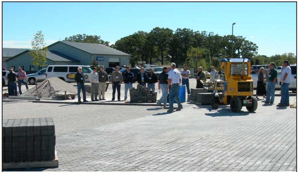
In the above photograph, the class just watched a demonstration of screeding the bedding layer, and is watching as I explain the layout, and the fundamentals of using the PaverMAX during mechanical installation.
