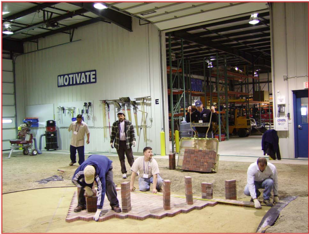
The latest Team Teaching class as they install pavers in the Best Practices method.
